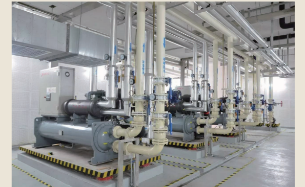
合肥万象城冰场制冷机房
